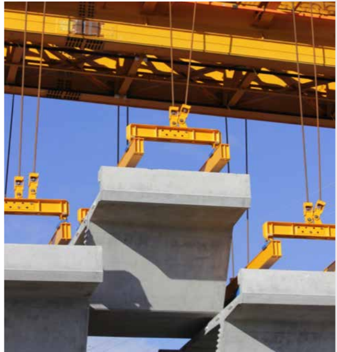
Traffic is stopped or detoured as each segment is lifted up to the launching truss with a winch. Once the four high strength steel bars are attached to the segments it is safe for vehicles to travel below.
